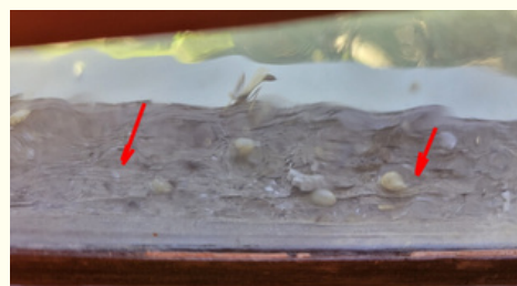
Looking through the glass of central "Christ" window - woodwork in need of repair & replacement.
